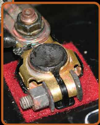
Battery terminal after BG Battery Service.
