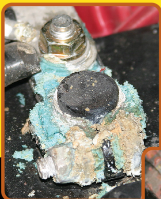
Battery terminal with corrosion buildup.
